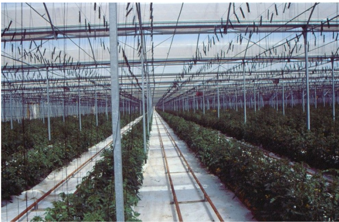
Figure 3. Internal view of a modern plastic 'Dutch' style greenhouse in the Murcia area of Spain (Duran Brothers). Tomatoes are grown using hydroponic culture, bumblebees for pollination, and additional heat in winter months.
